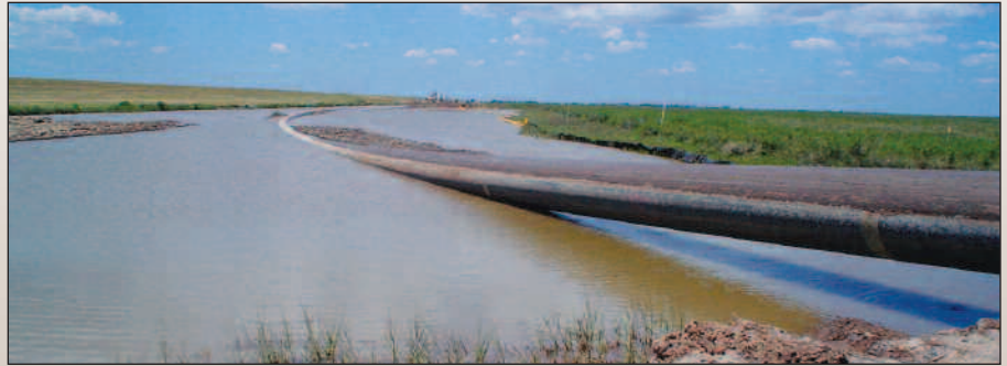
The approximate 5,000-ft tailpipe was floated in a borrow ditch dug in an existing canal adjacent to the wetlands marsh exit hole.
