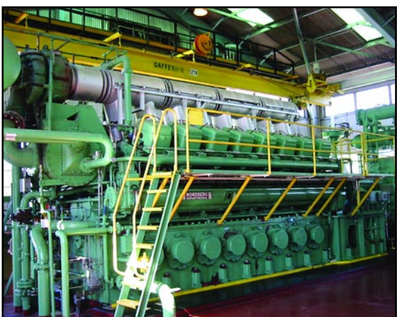
Figure 3. Gas-fired engine driving centrifugal compressor (background)
