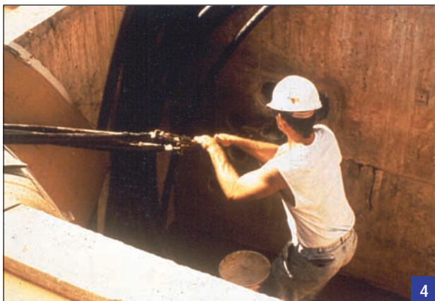
Underground duct system.
