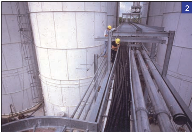
Cable tray system.
