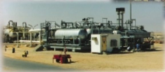
Onshore Flow Station
