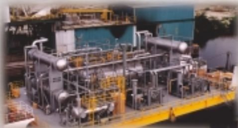
Offshore Oil Heating and Separation Module
