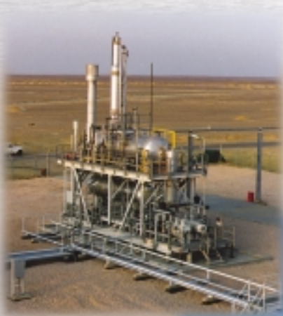
Onshore Sour Gas TEG Regeneration Unit
