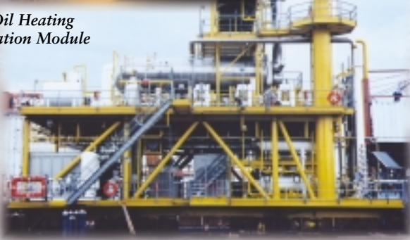
Offshore Gas Sweetening and Dehydration Module
