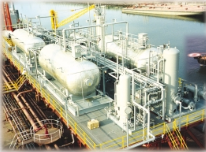
Oil Treating and Desalting System for FPSO
