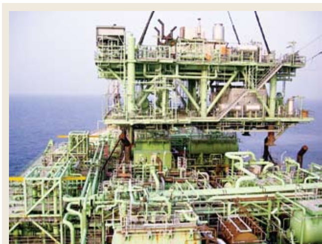
Fig. 2. On large offshore platforms and FPSOs the original design and piping drawings can often be missing or incorrect.
