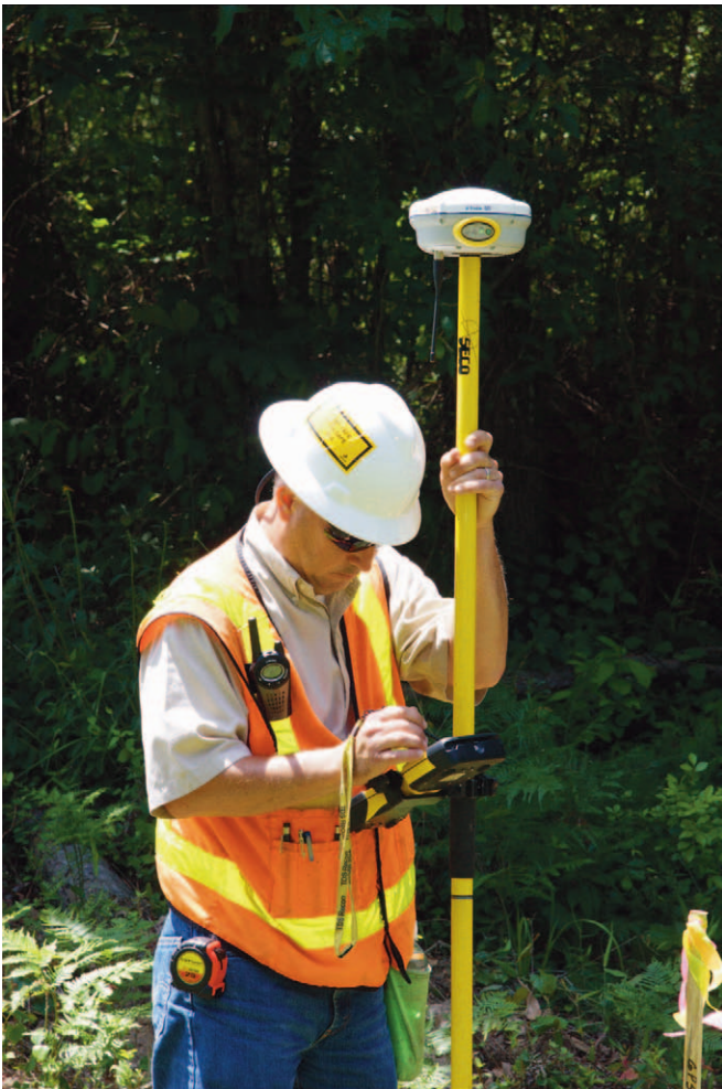
Figure 3. Survey teams stake land tract unit boundaries as well as access roads and the drilling well pad.
