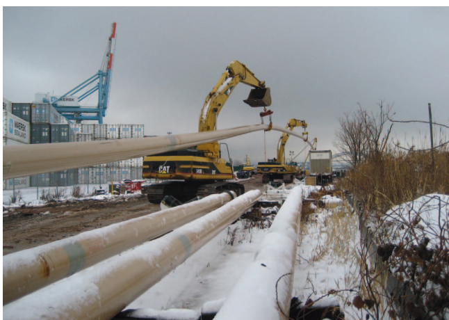
Figure 4. Rights-of-way can be in congested regions, requiring ingenuity to create suitable work areas.
